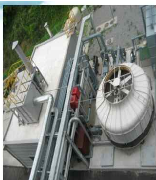
Utility & Cooling tower
